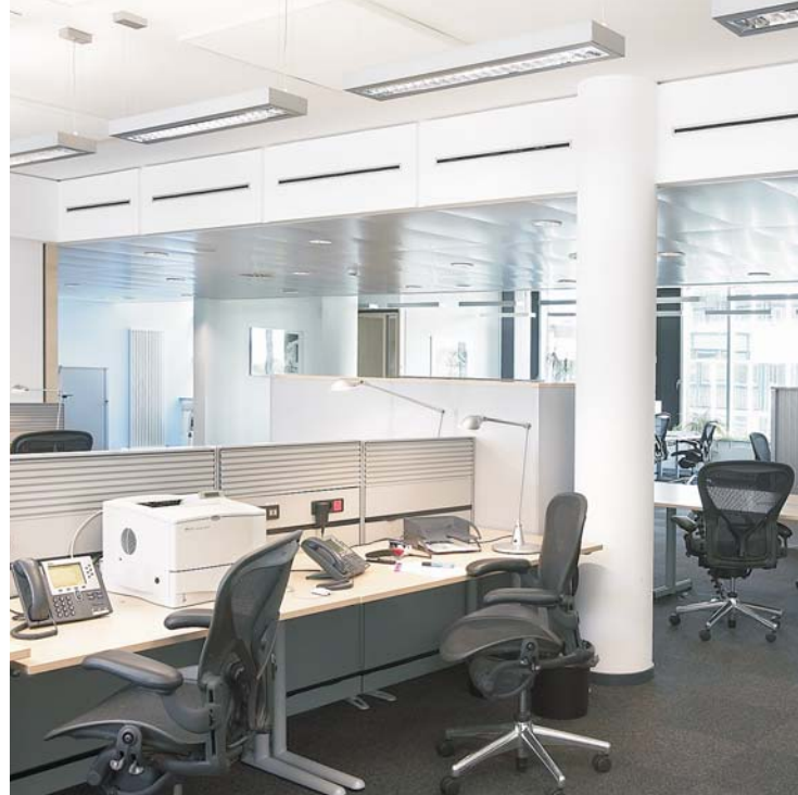
Wall slot diffuser, type WSD, in an office building of Mercer Oliver Wyman, Frankfurt am Main / D
