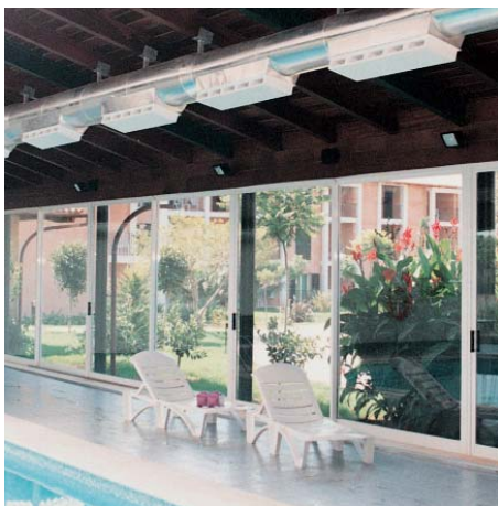
Linear whirl outlets, type WL, in the swimming pool of a hotel on Majorca / E
