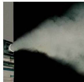
Air jet pattern of SW Jet slightly inclined upwards (Cooling mode)
