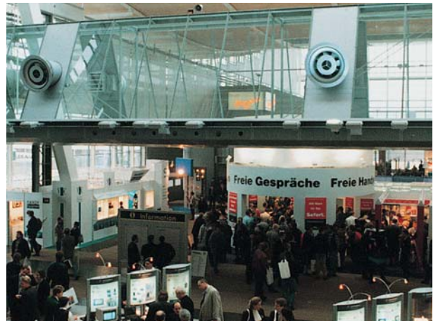
Swivel jet outlets, type SW, in the glass supply air duct, Hall 26, at Hanover Fairgrounds / D
