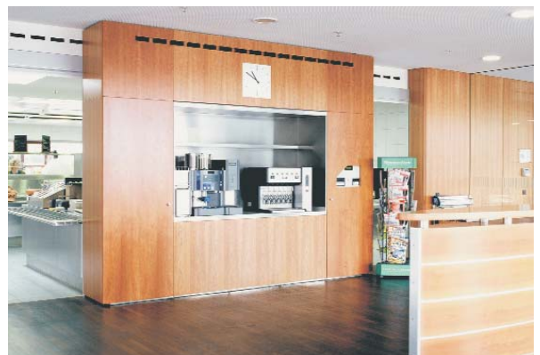
Linear whirl outlet, type WL, in the canteen of the Bavarian Office for Environmental Protection in Augsburg / D
